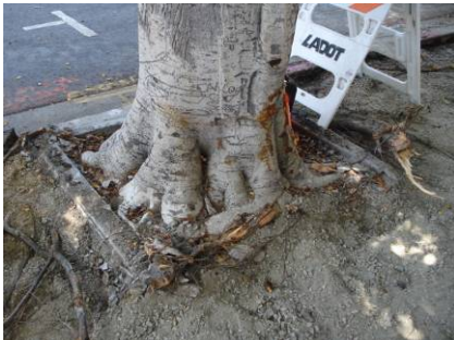
Tree that has outgrown original concrete tree well, now too small
